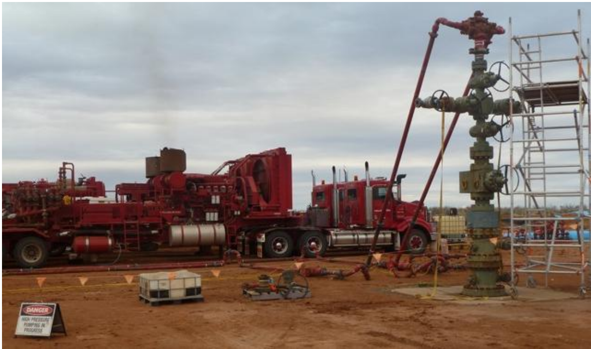
Figure 1 Some of the 8500 horsepower of pumping equipment utilized during the fracture stimulation
